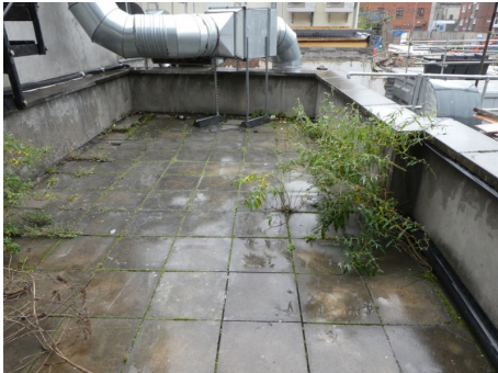
View of foliage growth noted on the rear elevation roof terrace
