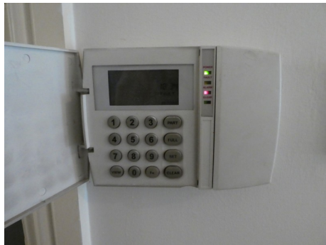
Typical view of a faulty security alarm control panel
