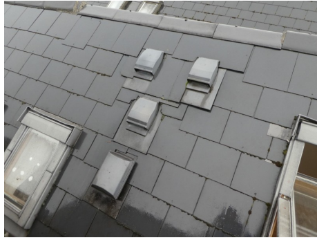
View of a small number of slipped and cracked artificial roof slates over the main roof
