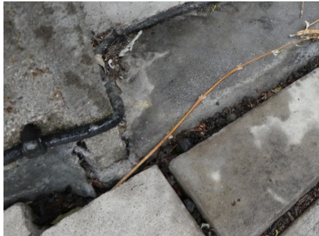
View of the poor flashing/weathering detail noted at the junction of the first floor rear elevation door threshold and roof terrace
