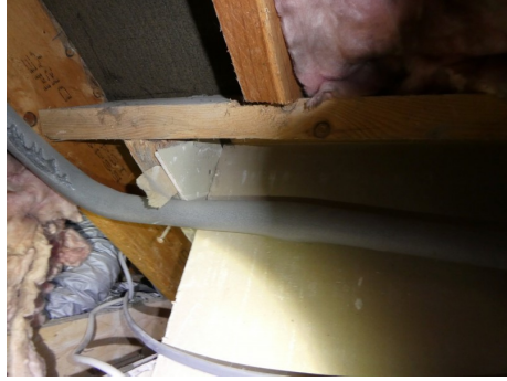
View of inadequate timber trimmers adjacent to a roof light within the roof space
