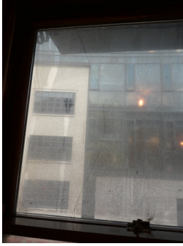
View of a cracked first floor window pane
