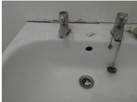
View of a cracked and defective wash hand basin
