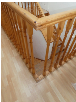
View of the loose and defective balustrade noted to the top floor
