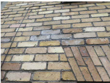
View of efflorescent salt staining noted to the front elevation brickwork
