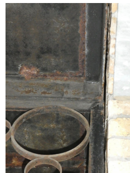
Typical view of a corroding external metal balcony deck
