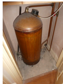
Typical view of of an uninsulated and inefficient hot water cylinder
