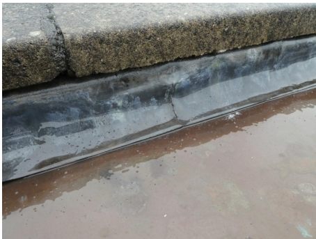
View of a cracked Lead flashing over the main roof parapet gutter; also illustrating contact between the Lead and copper where there is a bimetallic corrosion risk
