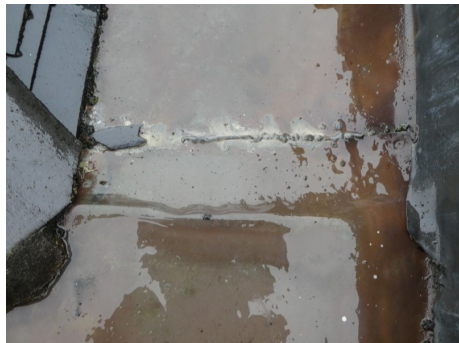
Typical view of a welded copper lining within the main roof parapet gutter which we suspect will have a limited life
